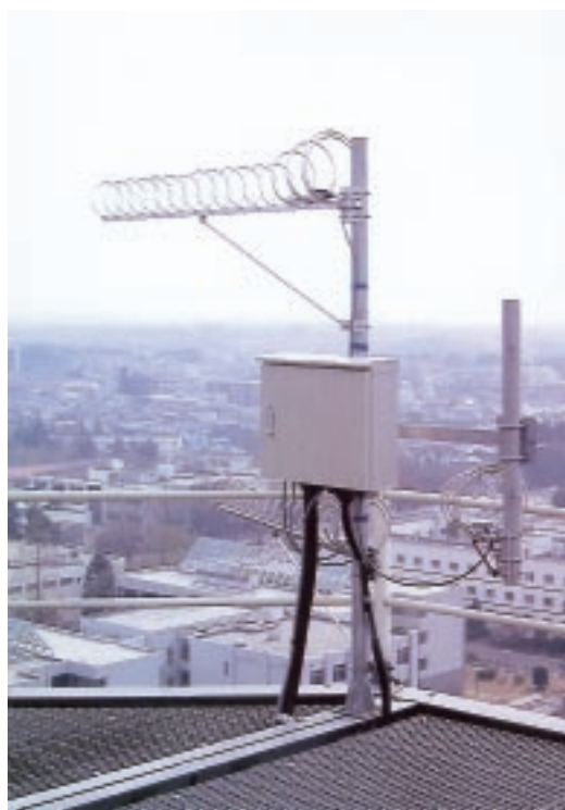
Digital terrestrial broadcasting antenna for experimental purposes
