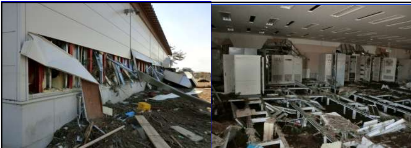
Sendai East Submarine Cable Landing Station
