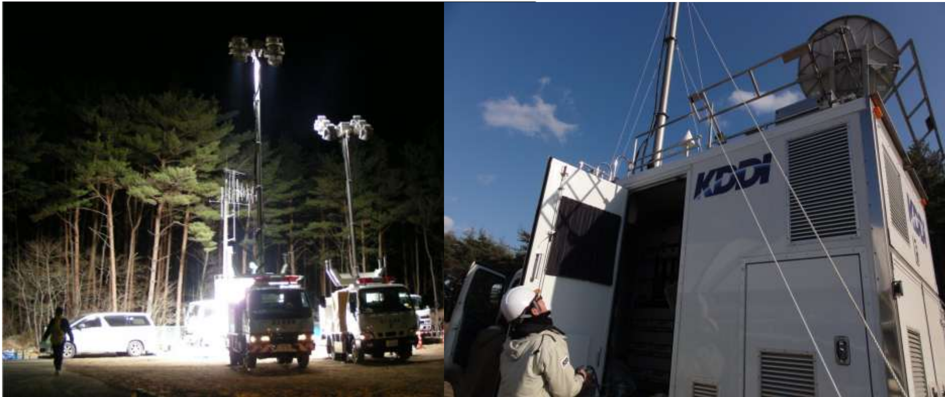
Mobile base station
