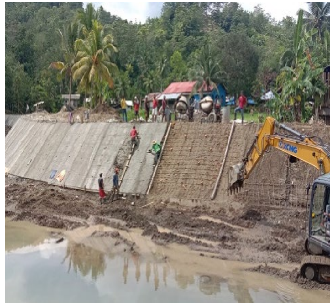
Construction of Flood Control System at Buayan River, Kabalasan, Zamboanga Sibugay under LGSF-FALGU
