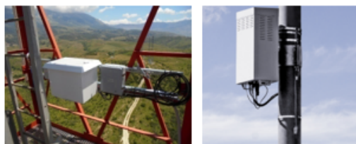
Typical modern integrated radio spectrum monitoring station 44
